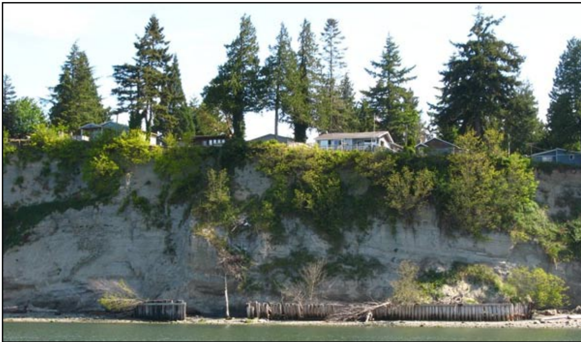
Figure 12: Vulnerable Homes on Hermosa Point
