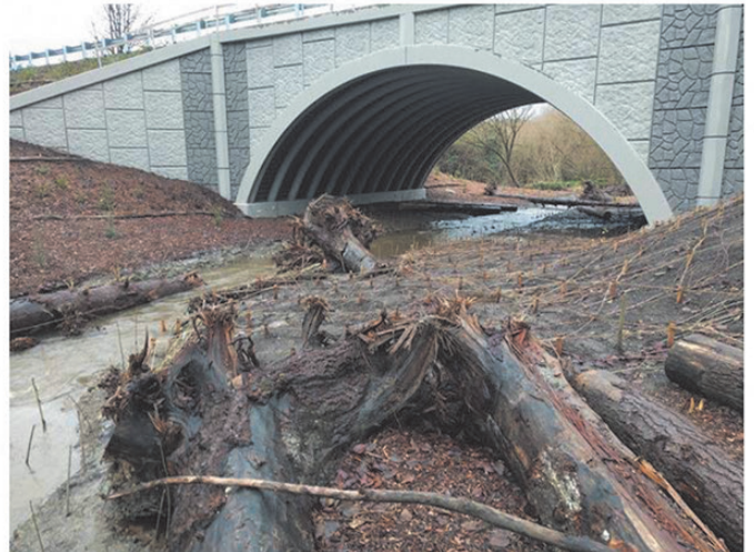
Culvert replacement of a 60-inch barrier culvert on Loutsis Creek on the Snoqualmie River
