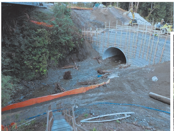
Replacement of a barrier culvert on Trafton Creek on the Stillaguamish River.
