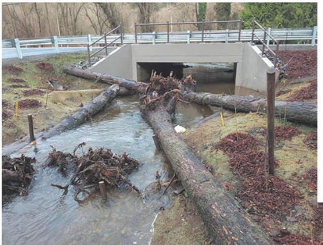
Replacement of culverts on Patterson Creek on the Snoqualmie that were barriers.
