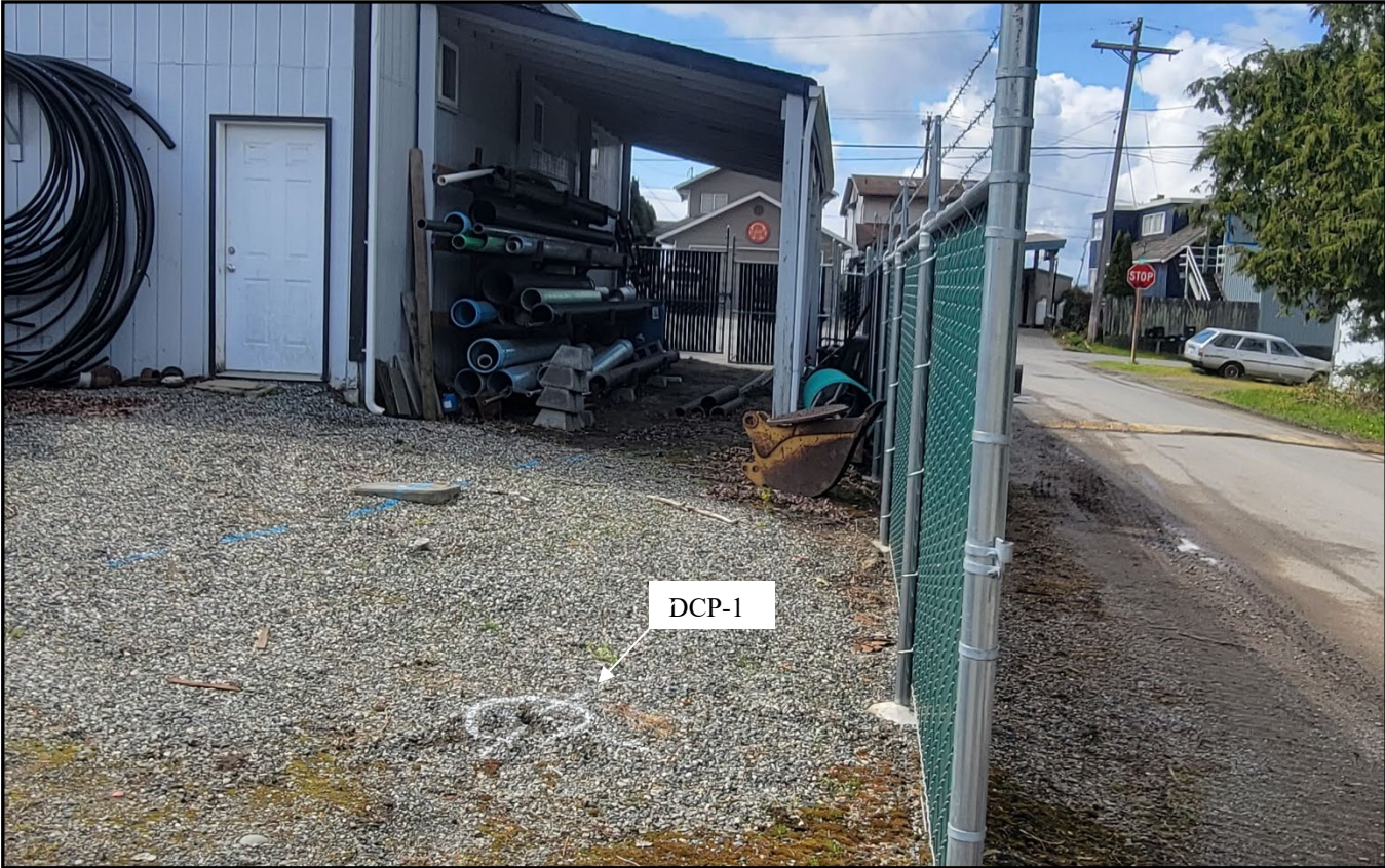
Photo A: Looking south at the northwest corner of the building. DCP-1 in progress
